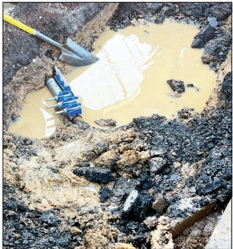
Thanks to Gladewater interim city manager Charlie Smith the year-old water leak at Loop 485 and US 80 is now fixed. The city's former city manager told the Mirror TxDOT would not allow the city to fix the constant leak, because it is on a state highway. But after a call to TxDOT by Smith, city and TxDOT crews were fixing the leak Monday morning.
