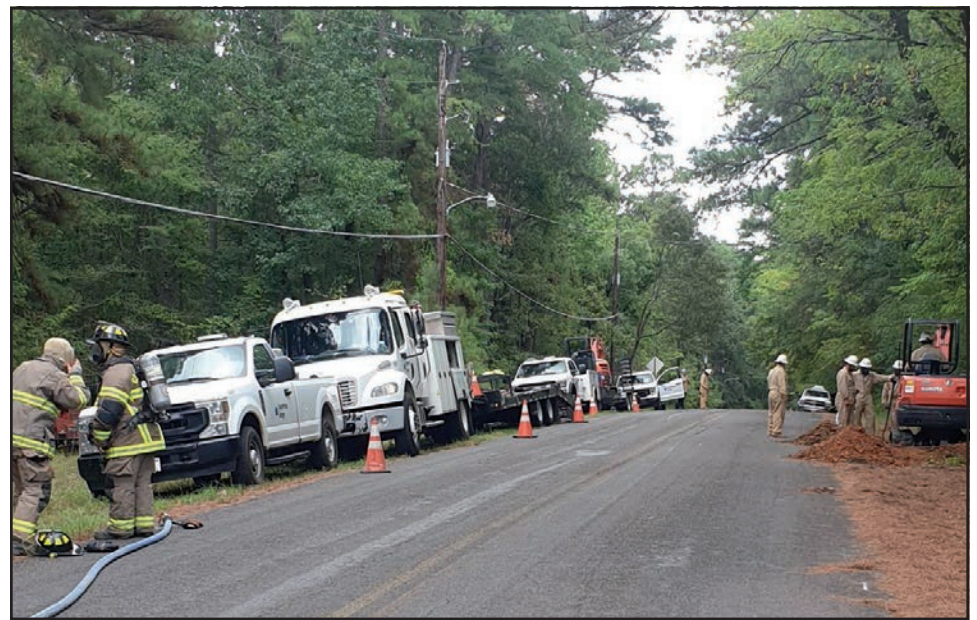
A gas line that contract crews hit while boring last week resulted in a partial, neighborhood evacuation. Gladewater firefighters were on the scene and worked quickly to locate the source area of the leak, clear the area, block roadways and evacuated about 15 homes for safety. GPD as well as Public Works helped with road closures and blocking. Centerpoint was able to locate and cap the line then continue on to make the final repair.
