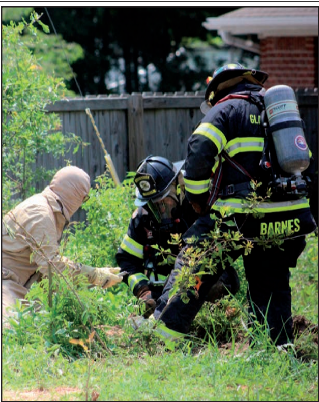
Gladewater Fire Department's Aaron Brandt and Shane Barnes assist CenterPoint Energy's Clayton Myers in re-plugging an exposed gas line in the 2100 block of E. Broadway Ave. shortly after noon June 8. The quick re-seal took just minutes after the valve was bumped by a construction crew. Photo by James Draper
