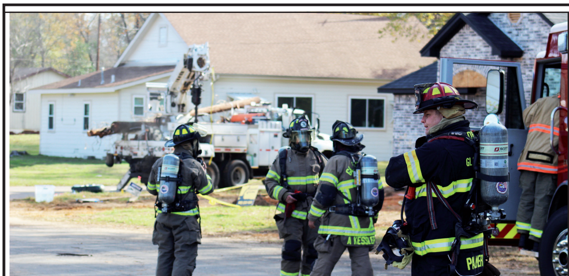
Gas escapes from a borehole at a Roden Lane construction site Dec. 6 after a utility crew punctured a four-inch lane in the residential neighborhood. Gladewater firefighters controlled the scene and issued shelter-in-place orders until CenterPoint Energy personnel could arrive and get the leak under control. Photo by James Draper
