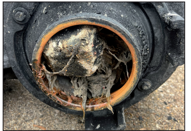
A brick clogs one of the City of Gladewater's lift station pumps in mid-December 2023, necessitating yet another time-consuming and costly repair.
