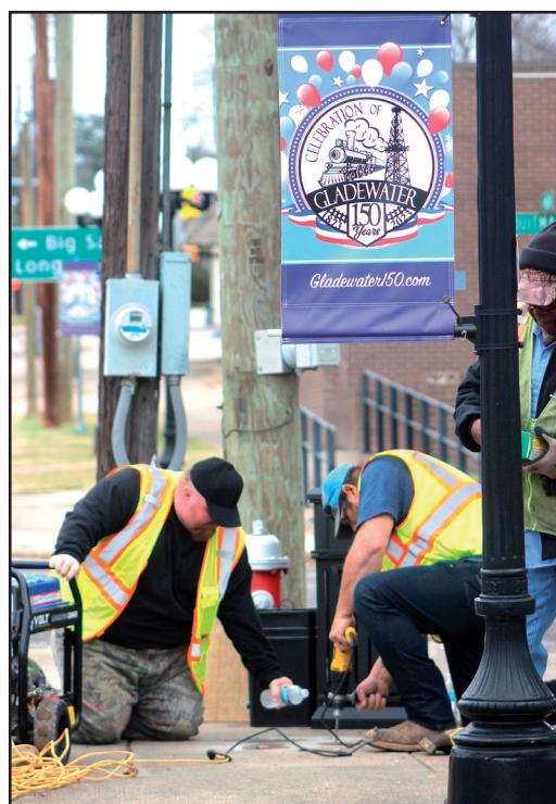
Gladewater Public Works employees install one of downtown's new trash containers Monday morning. About 15 of 20 units have been replaced so far in one of the department's first projects of 2024.
