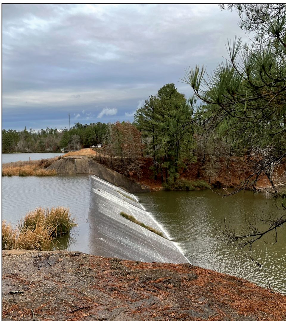
Recent rainfall has raised the level of Lake Gladewater enough for a healthy run-off over the concrete spillway. The most recent annual inspection of the dam puts it in ‘poor’ condition as the City of Gladewater works toward consistent maintenance and improvement while pursuing grant-funded repairs.
