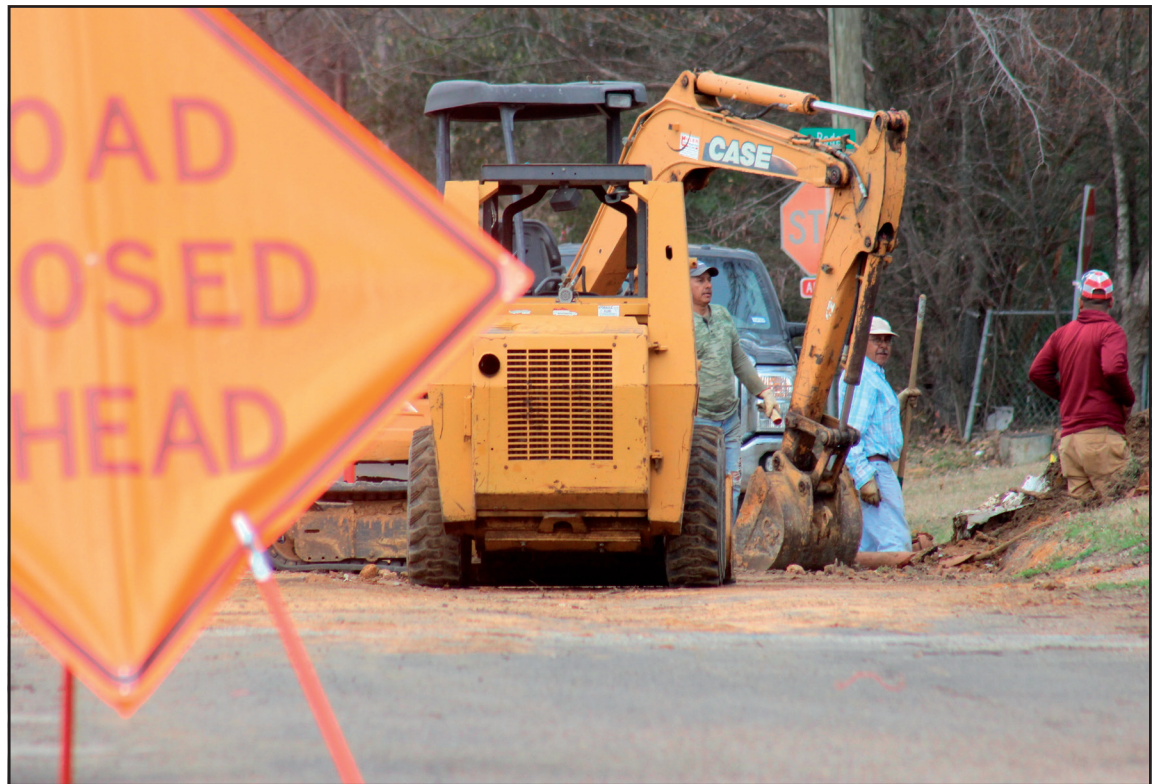
A crew works on Hendrix Friday, one of numerous Public Works projects active across the city amid an array of water leak repairs and other tasks. Photo by James Draper
