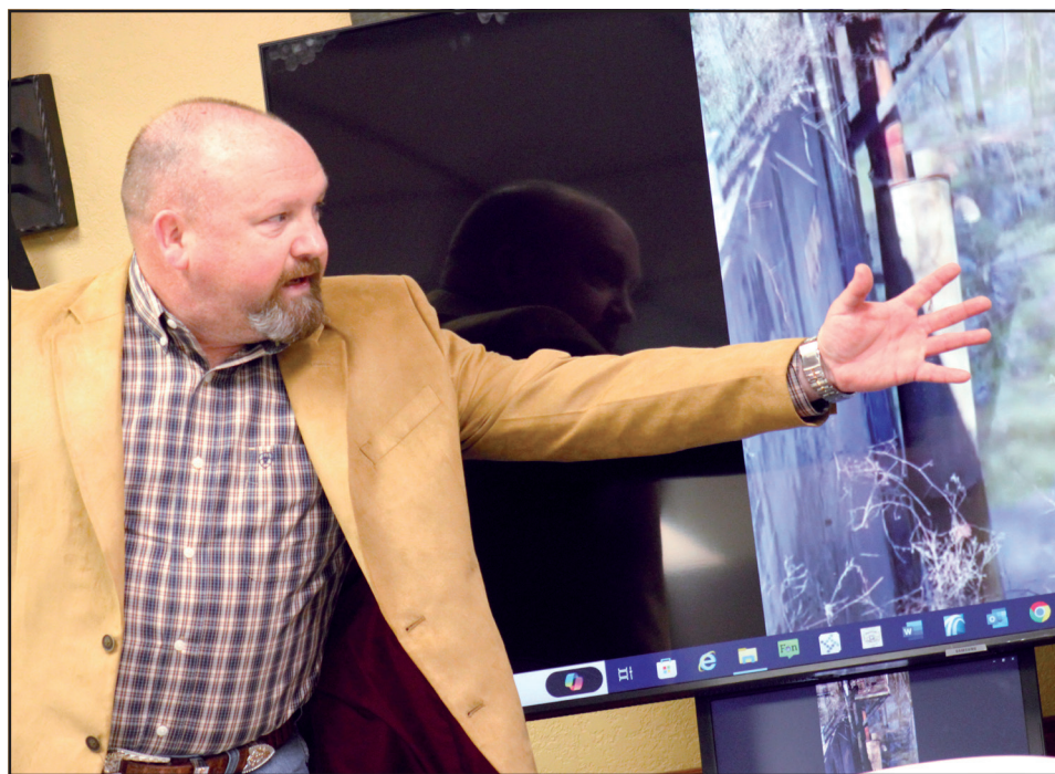
White Oak City Coordinator Jimmy Purcell points out the problematic tilt in the 'can' at the community's water intake on Big Sandy Creek. A careful repair is necessary and could reach as much as $100,000 if the equipment fails any further.
