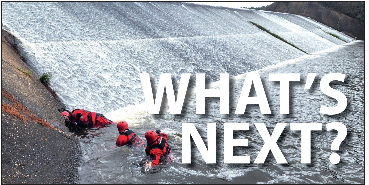
Gladewater Fire Department Driver/Operator Aaron Brandt puts his head in a void large void in the concrete spillway at the Lake Gladewater Dam, joining Fire Chief Mike Simmons, SPI Engineer Andrew Wright and GFD Driver/Operator Stephanie Lopez on another up-close examination of the flawed structure Friday. Courtesy photo from Mike Simmons
