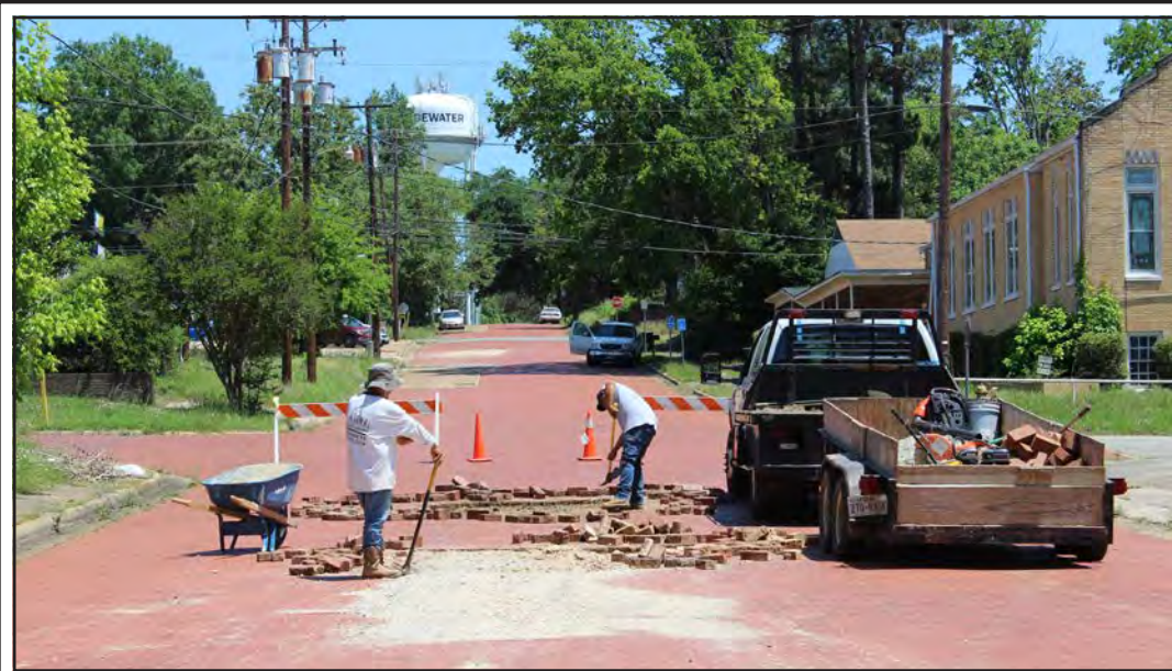
Center Street's historic red brick streets were under repair last week to return them to level heights and to their original brick design eliminating the patching done by city and utility crews after water and gas line breaks. Work has been completed on Quitman Street. The project is sponsored by the Gladewater Economic Development Corporation. Photo By Suzanne Bardwell
