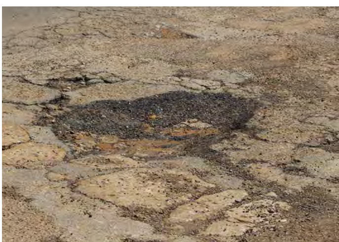
The harsh spring weather has played havoc with roads and streets. This pothole of the week is on Hendricks Street is just off Rodeo Drive.
