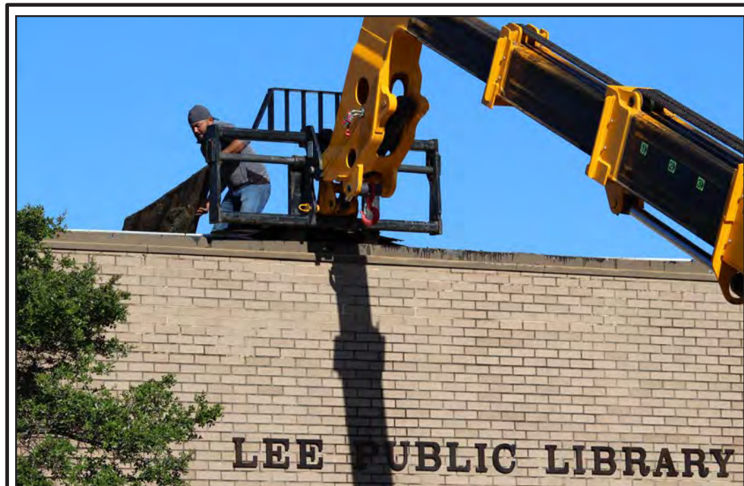
The Lee Public Library roof which was effectively destroyed in February's ice storm was being removed Monday. After removal a new roof will be constructed with a slight pitch which will improve the function of the roof. Paragon Roofing will be doing both parts of the roof project. The library interior has been completely redesigned by a Tocker Foundation library architect at no cost to the city to create a 21st century library/education/technology/job center.
