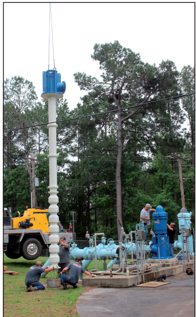
Crew members from Red River Pump Specialists and other contractors re-install Gladewater Water Plant pumps 2 and 3 Monday under the watchful eye of Plant Manager Wendy Emmel, Operator Nate Palmer and other city personnel. After a week's delay due to rain, the contractors went on to remove pump 1 for maintenance and a bit of TLC – it kept the city's water flowing on its own non-stop since the other pumps went out-of-service March 4.
