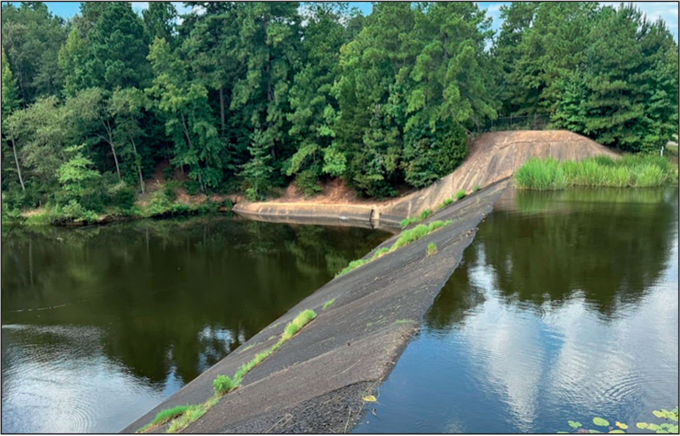
Now that annual inspections have resumed, City of Gladewater officials are tracking year-to-year deterioration of the concrete spillway portion of the Lake Gladewater Dam. (Below) Erosion has steepened the slope on the downstream side of the dam’s earthen embankment, requiring regular spraying to mitigation vegetation that could penetrating and weaken the 73-year-old structure. (Courtesy Photos by Mike Simmons)
