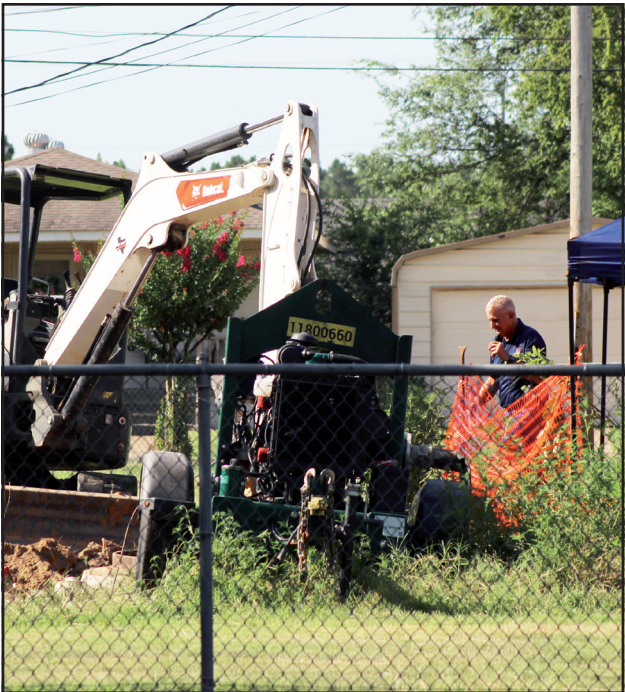
Gladewater Fire Chief Tim Basham gets a closer look at a leaking gas line July 29 after the mismarked equipment took a hit during an excavation project between residences on Eddy Street.
